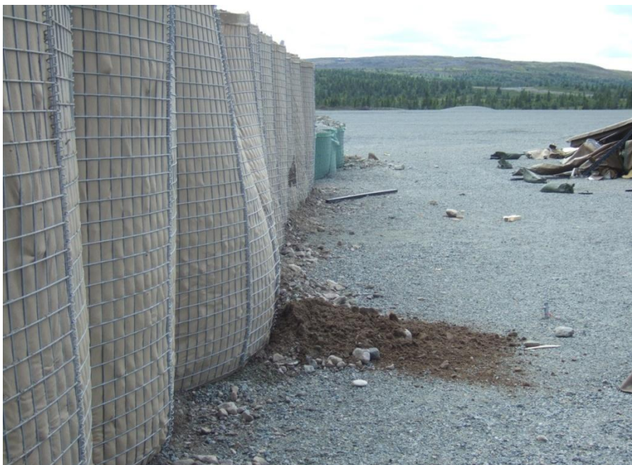
Figure 2.29 Back side of MIL 10 wall with local soil after detonation of a 155 mm grenade (test 1.14)
