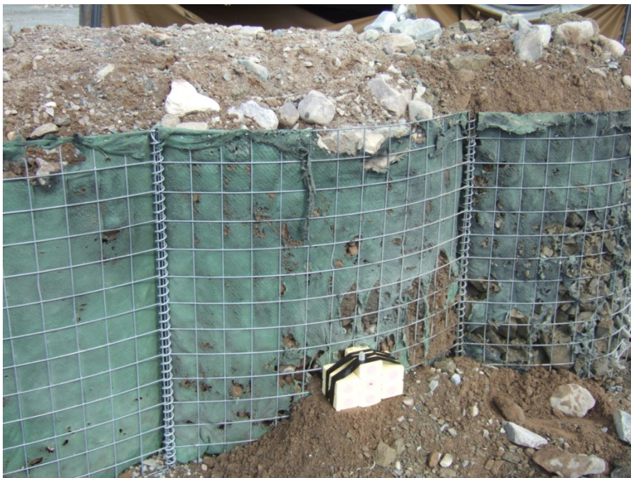
Figure 2.5 Setup of test 1.10 with 3.5 kg TNT at a MIL 3 wall with local soil
