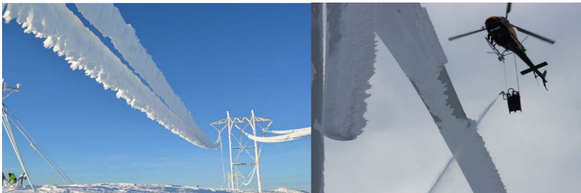
Figure 4.3 Icing on power lines and wind turbines is the subject of extensive research. The statistics and prediction tools are somewhat relevant to drones. (Left) The ICEBOX project has been working to increase knowledge about the icing process, ice shedding, and icing conditions statistics [22, 23]. (Right) De-icing wind turbine blades is a costly activity, but important, as ice shedding from wind turbines is a serious threat to safety (Image by Alpine Helicopter).
