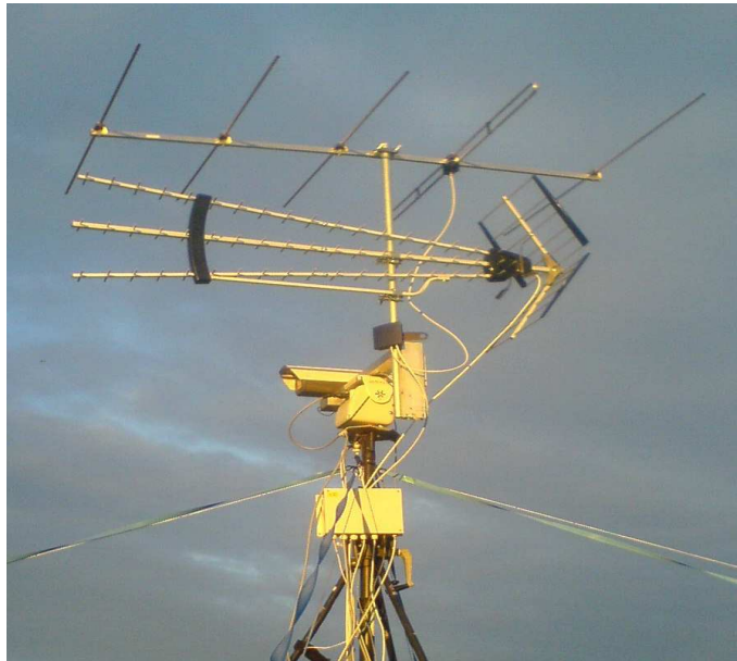
(a) Reference channel, FM radio antenna; TRIAX 5 element (upper antenna), DVB-T antenna; Televes DAT75 Digital Tv Aerial (lower antenna).
