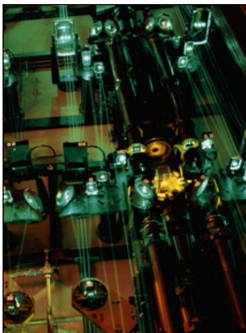
Figure 8.2 Laser corridor during AVLIS operation. Over 2000 optical elements convey these green and yellow beams. Each wall in the dye laser corridor has two dye laser chains, which amplify the light for later use in the separator tank. Special filters clean the air in the laser enclosures, making it 1000 times cleaner than that in a room with standard air conditioning. Photo courtesy of the United States Department of Energy.
